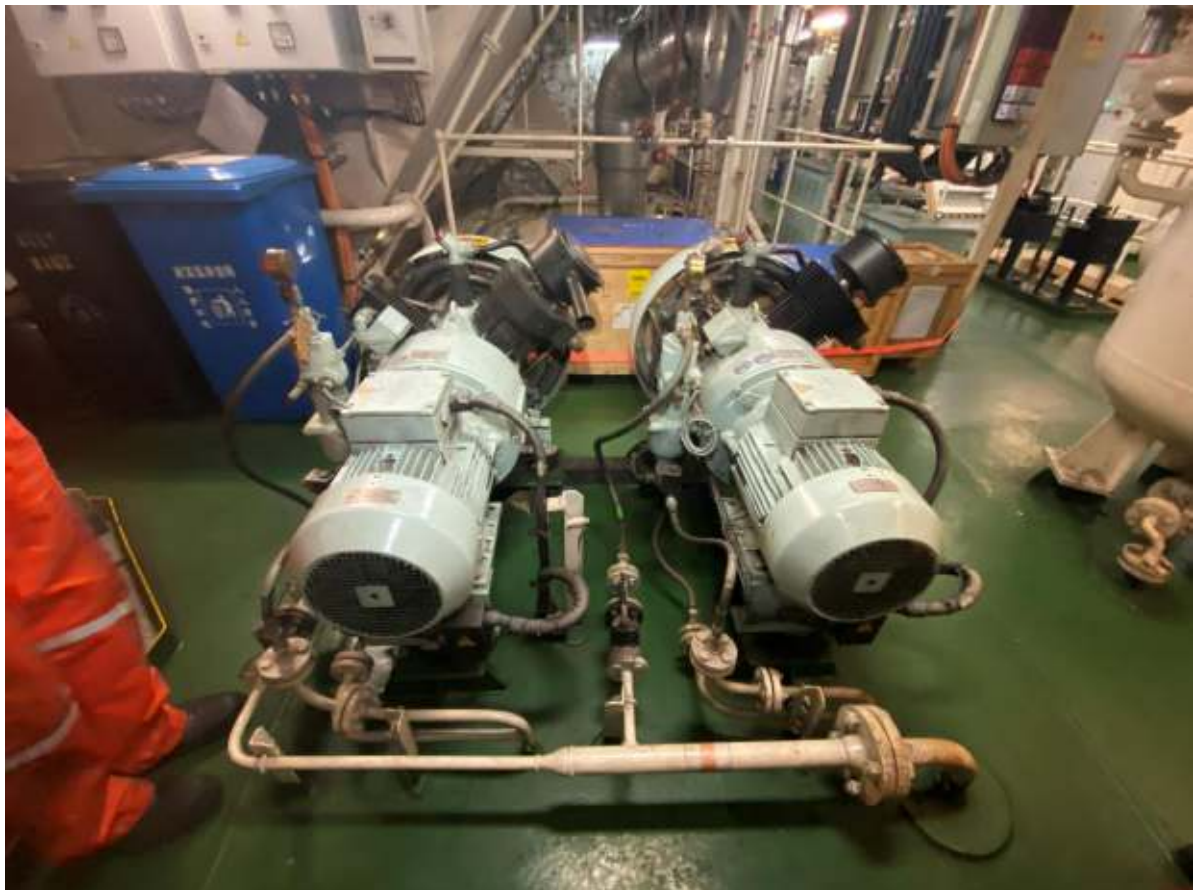
140. Main air compressor.
