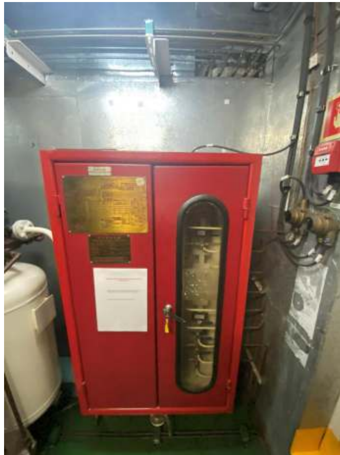
033. Quick closing valve cabinet.
