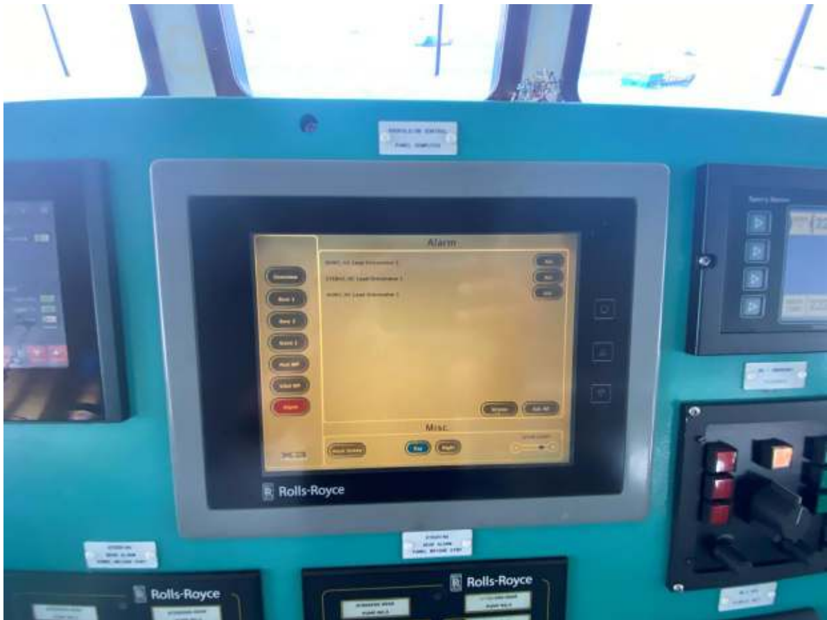
093. Propulsion alarm panel.
