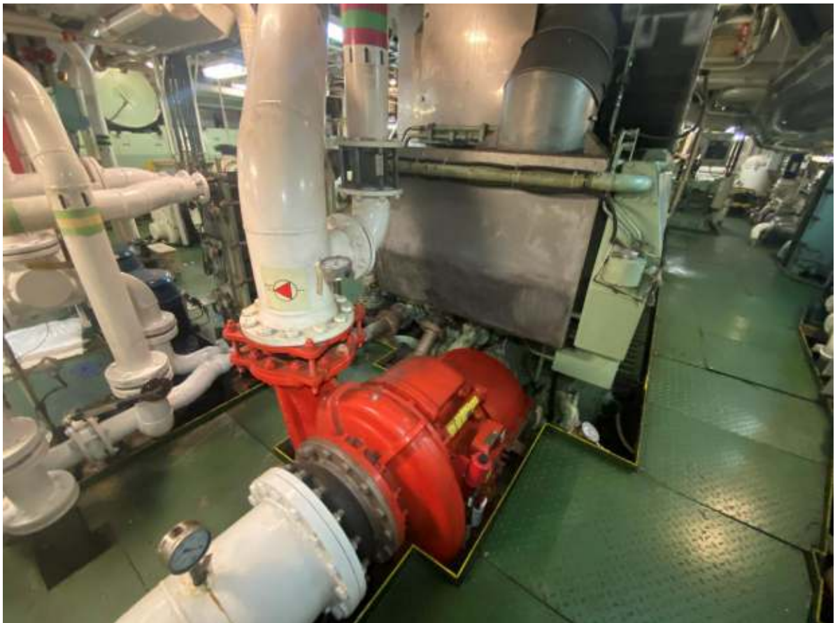
120. Attached FIFI pump no. 1
