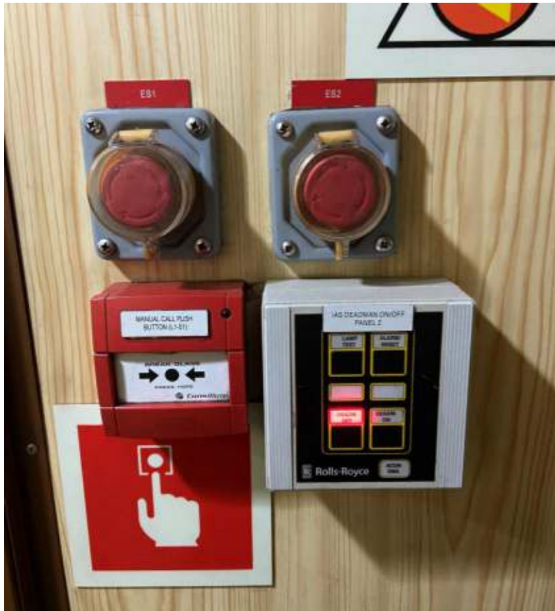
107. Dead man alarm outside of engine room entrance.
