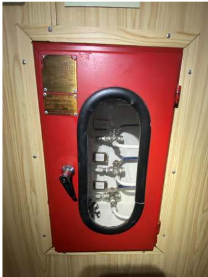
042. Quick closing valve cabinet.
