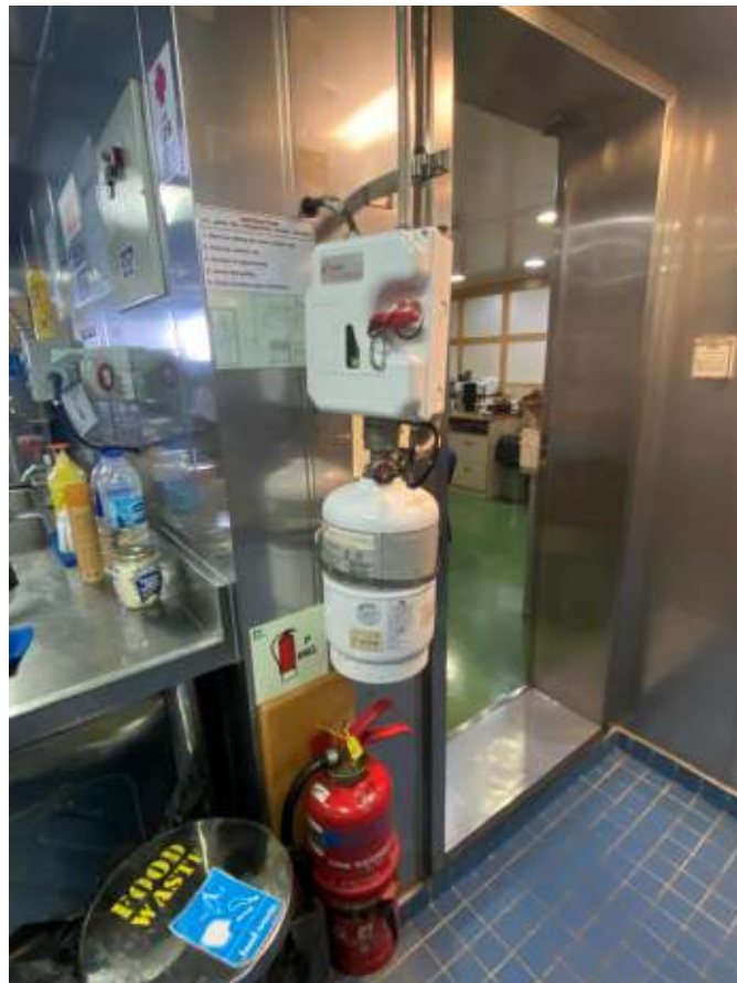
050. Chemical fire fighting installation.
