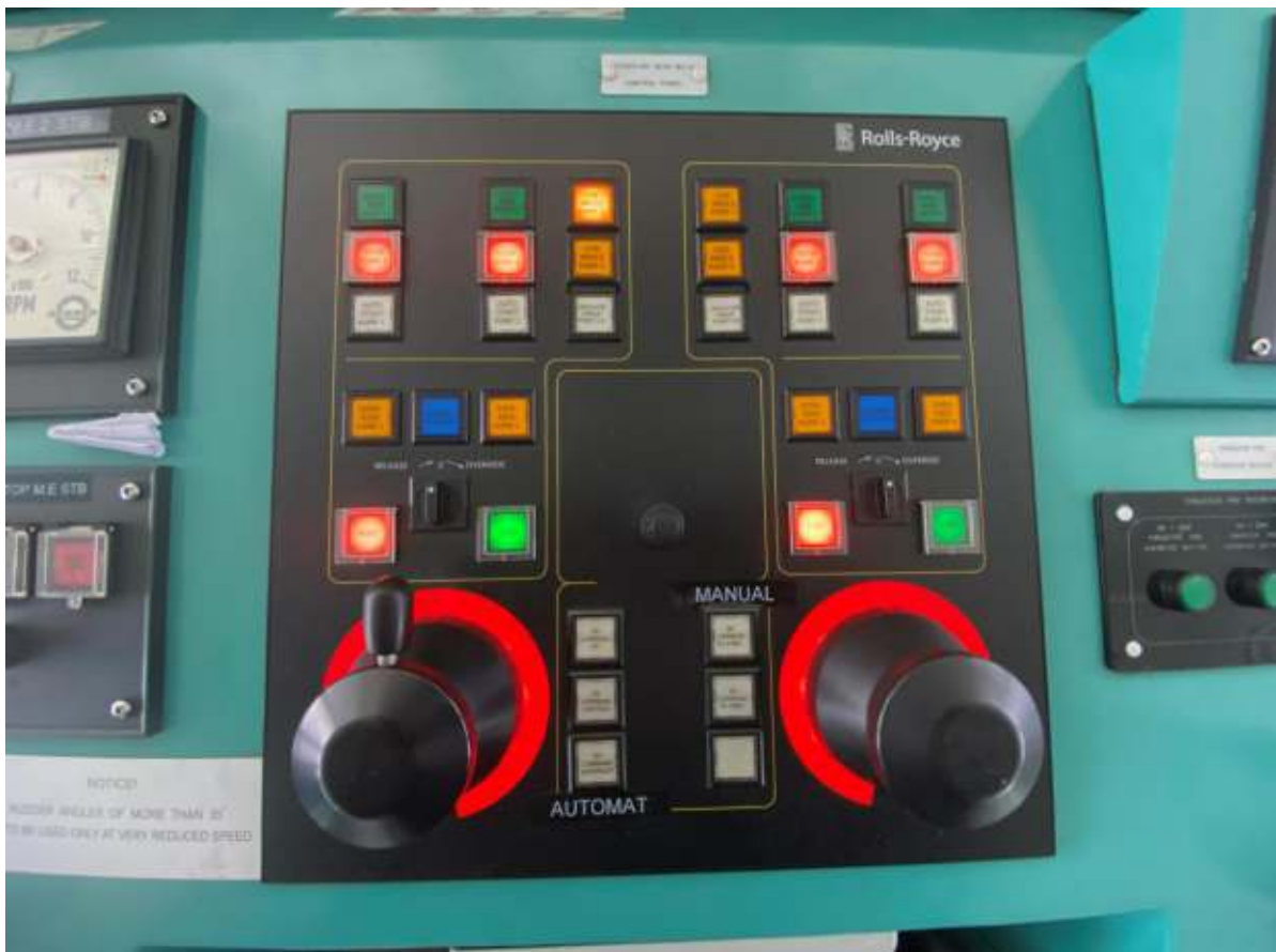
094. Steering gear main control panel.
