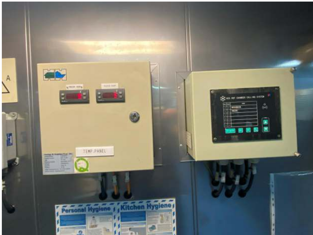
051. Freezer remote temperature display.
