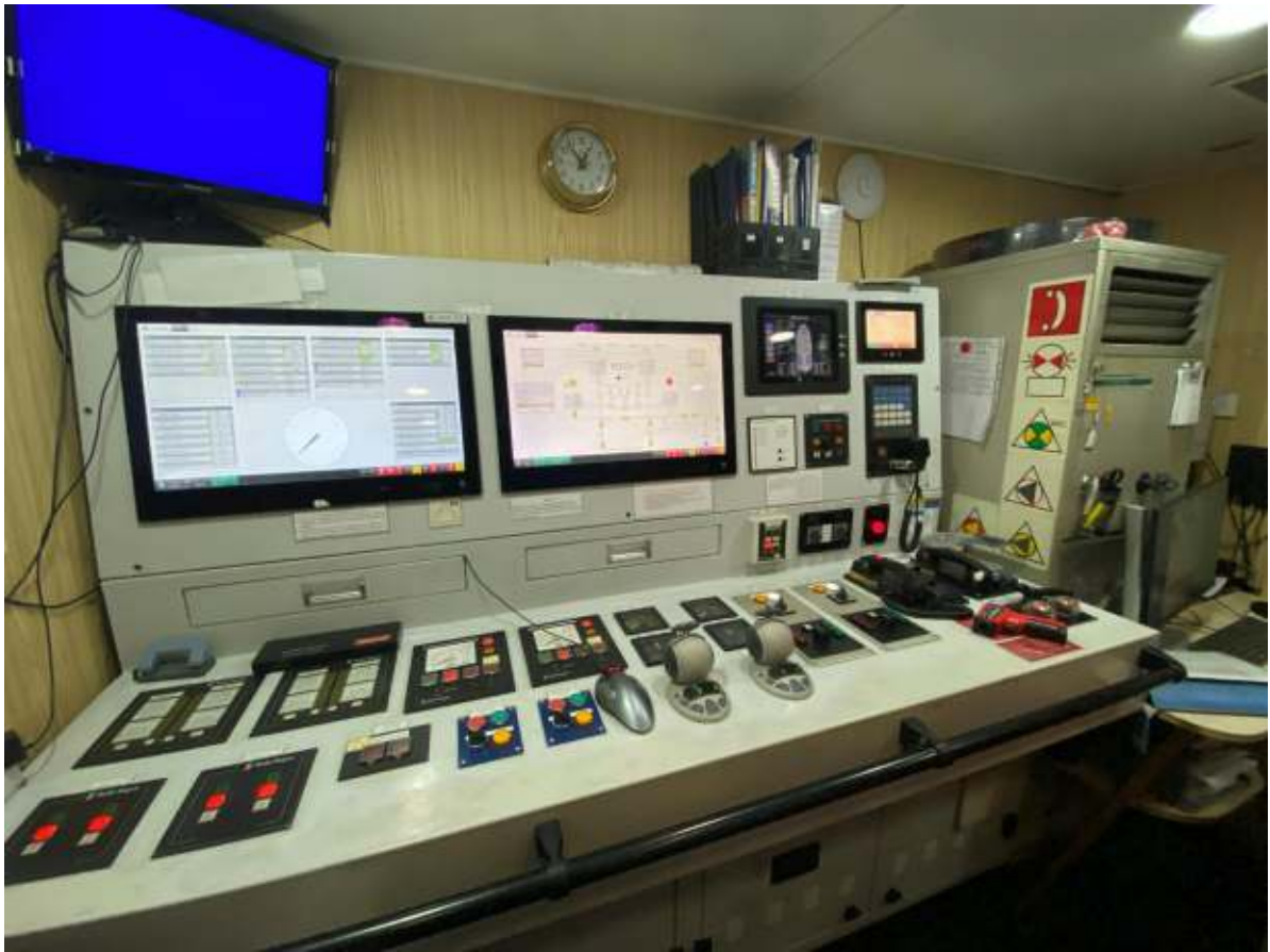
143. Engine room control console.
