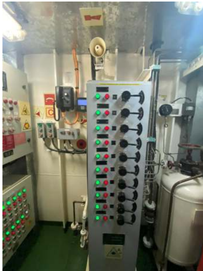
032. Water tight doors remote closing levers.
