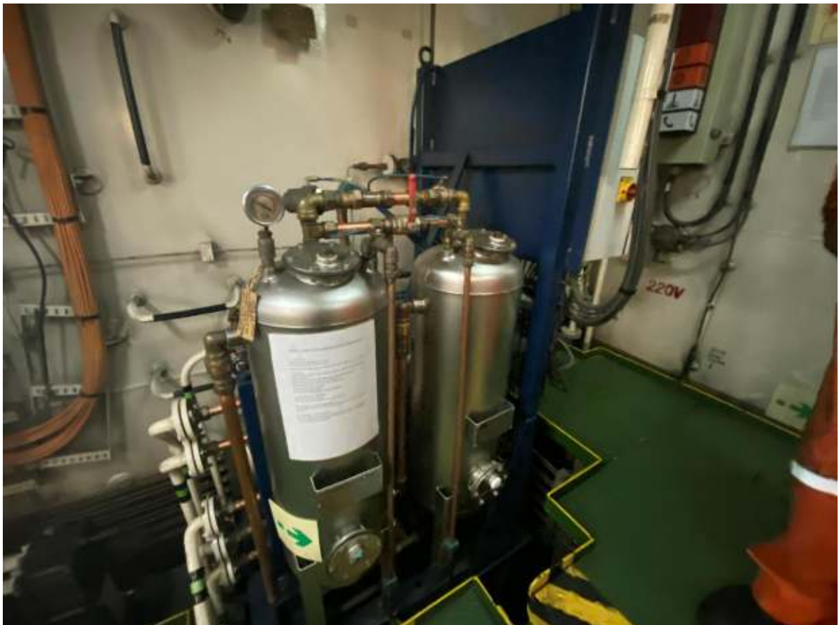
130. 15 ppm oily water separator.
