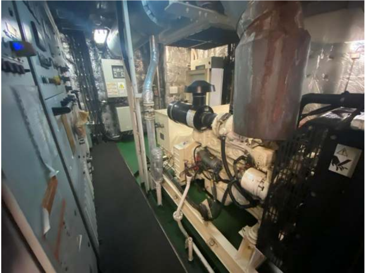
029. Emer. generator room.
