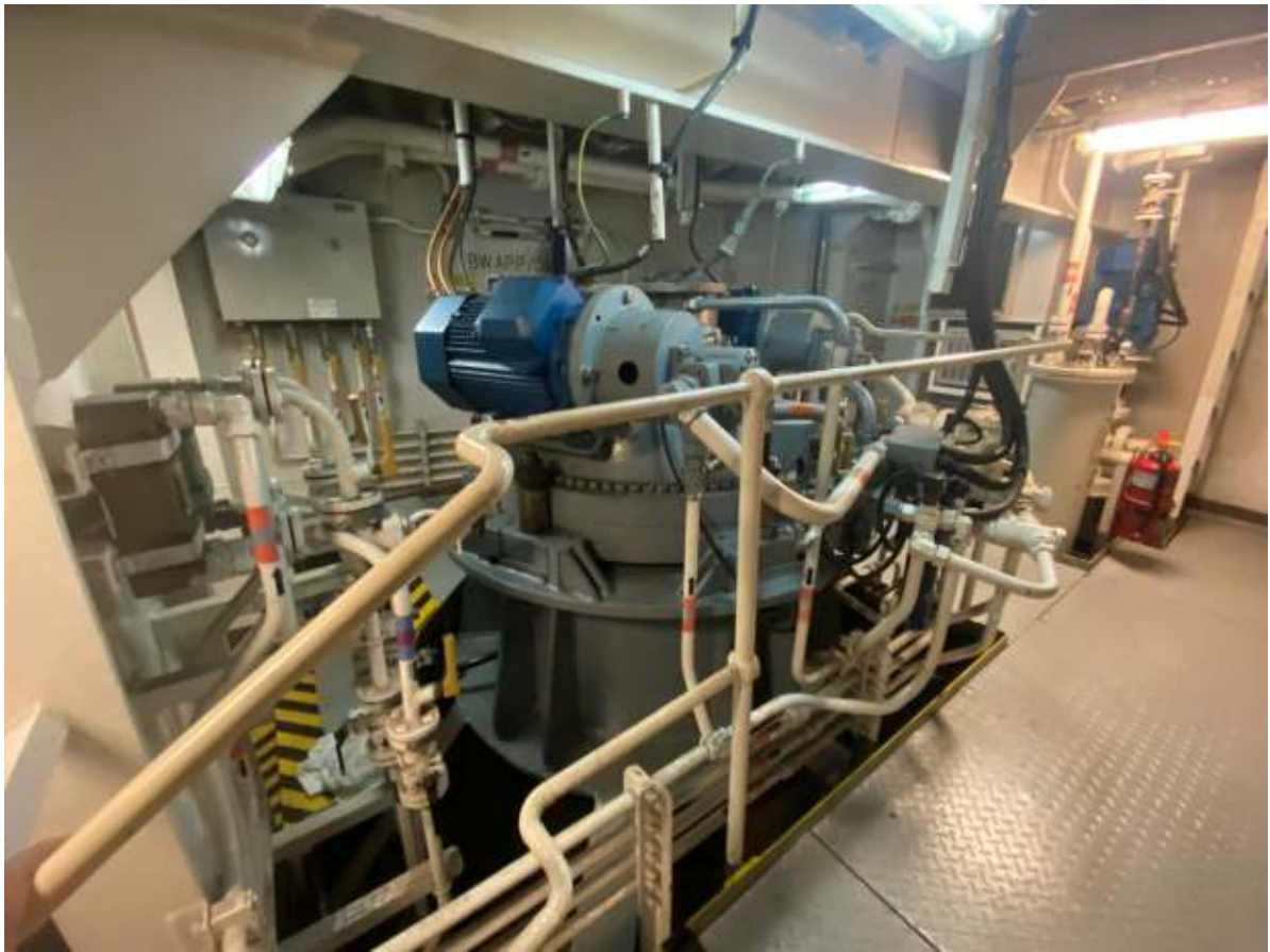
113. Portside CPP propulsion system.
