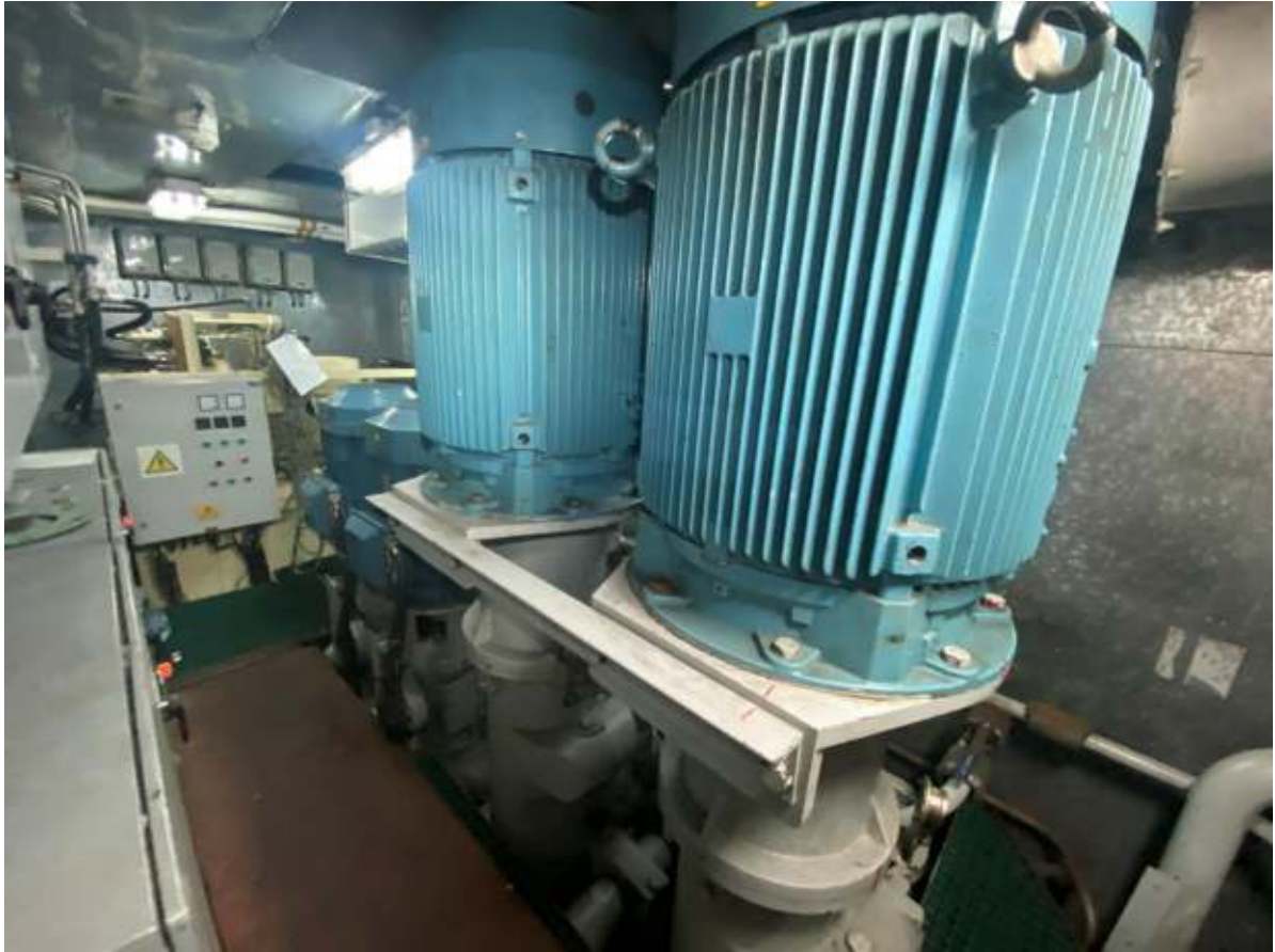
027. Hydraulic pack room.
