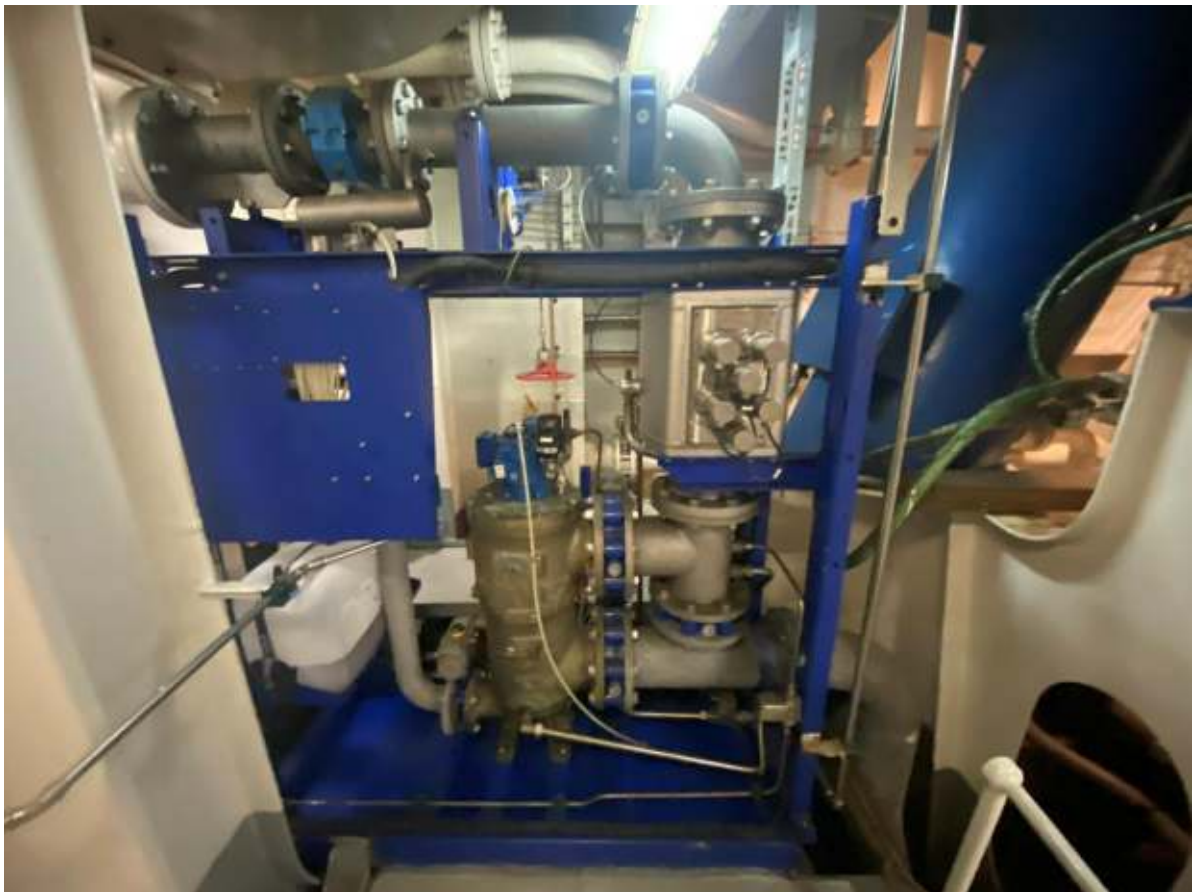
114. Ballast water management system.
