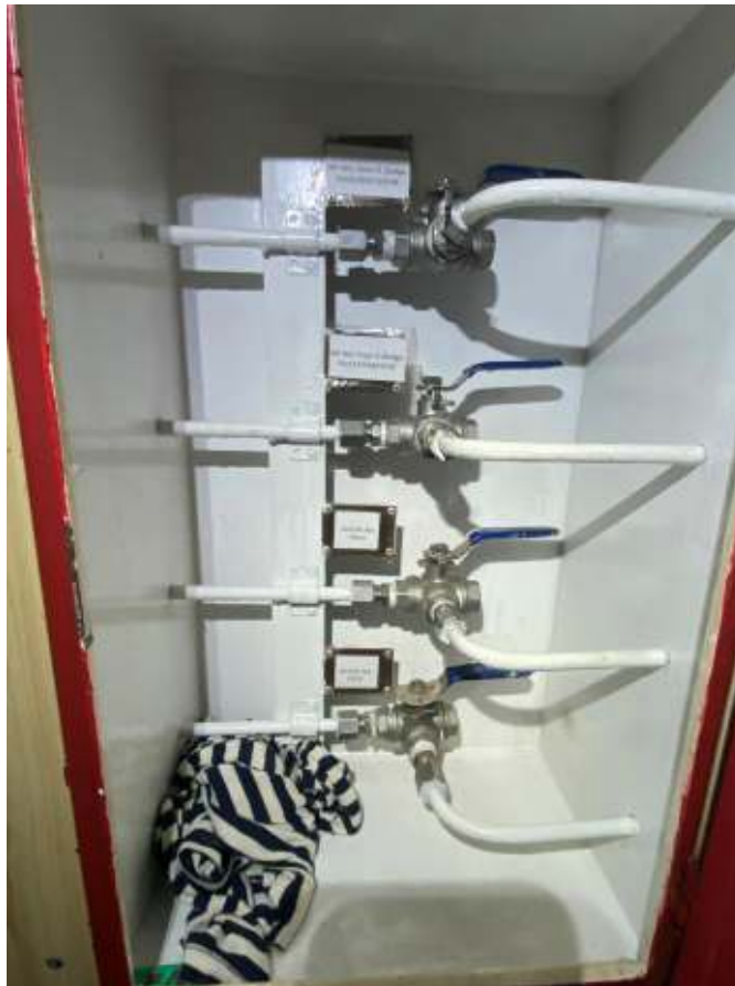
043. Quick closing activating valves for several machineries.
