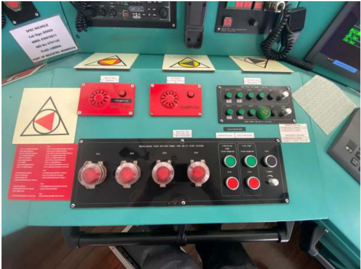
089. Emergency stop switches.
