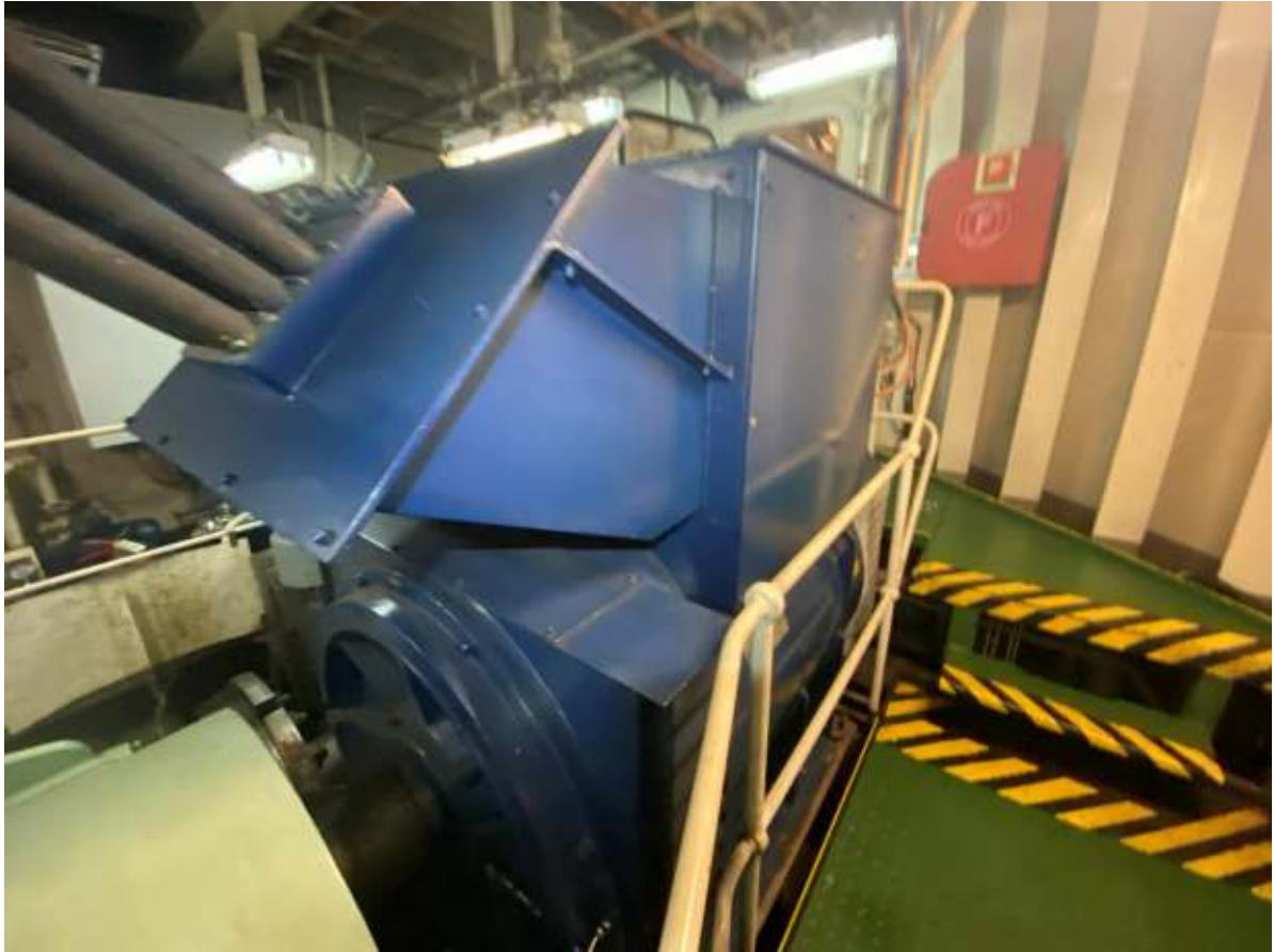
129. Electric propulsion motor.
