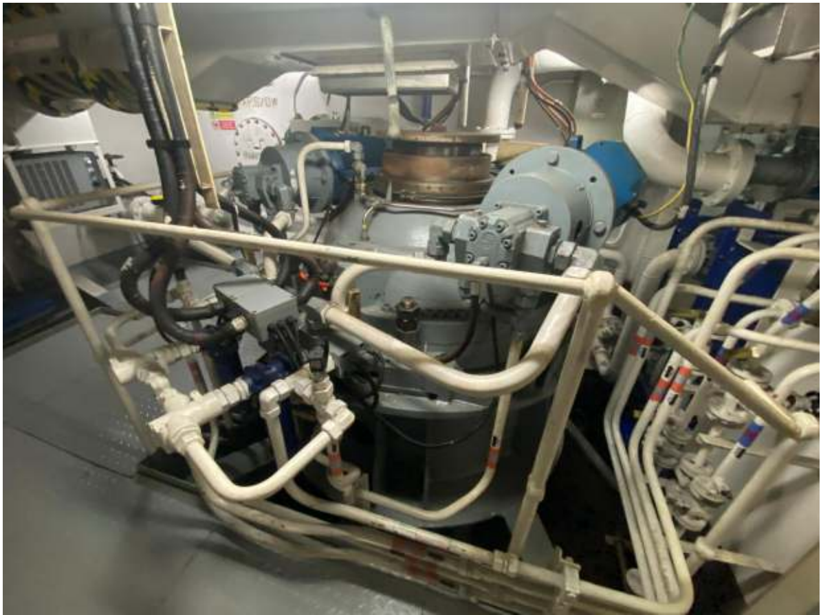
115. Starboard CPP propulsion system.
