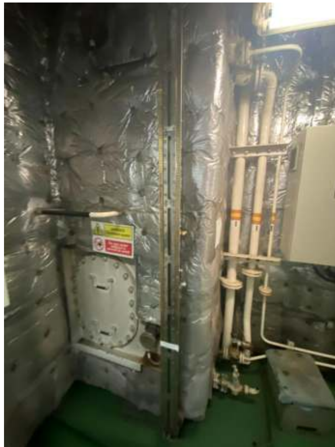
030. Emer generator fuel tank.
