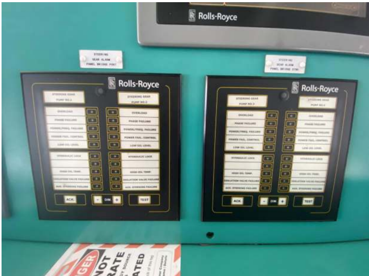
092. Steering gear alarm panels.
