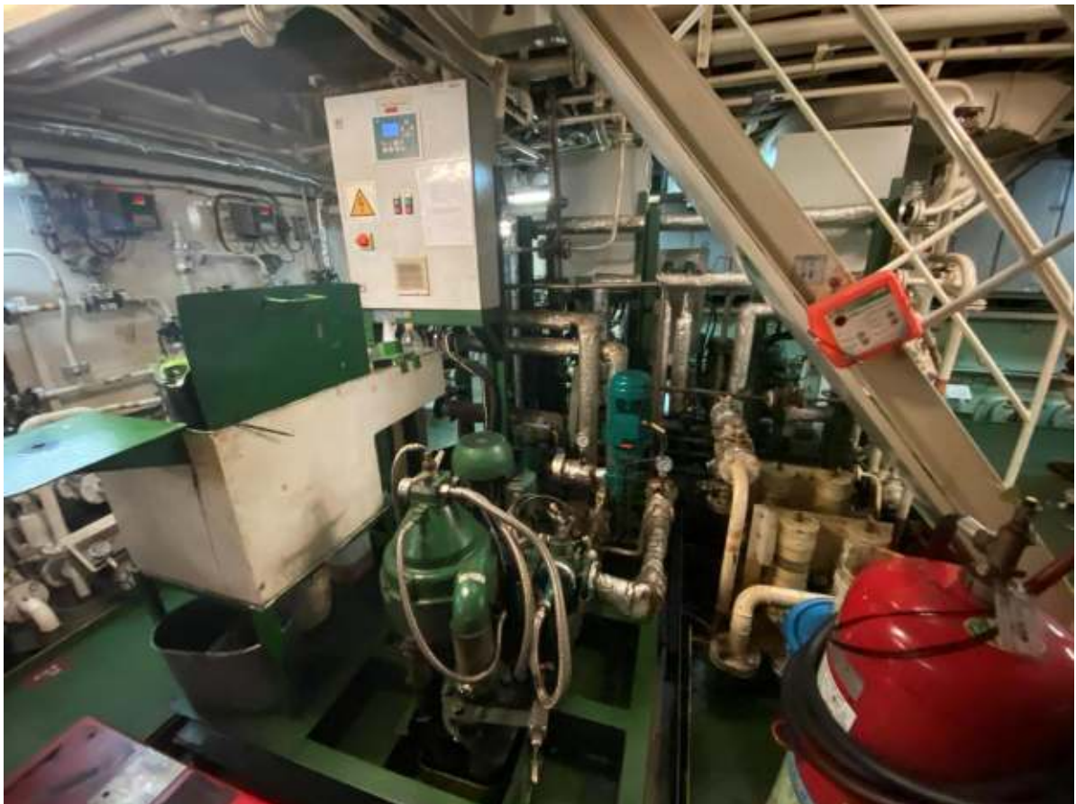
144. Diesel oil separator.
