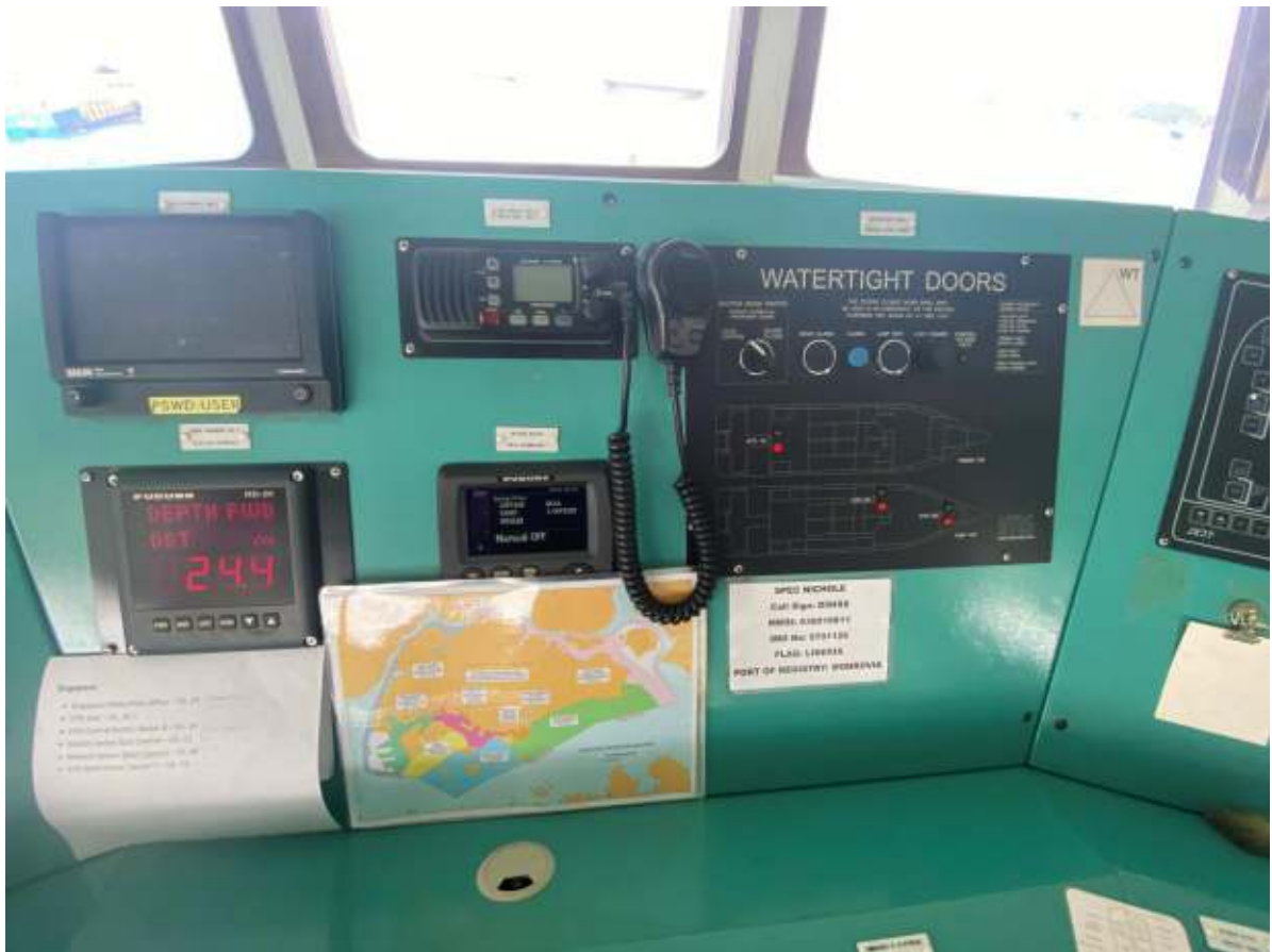
097. AIS, Bridge alarm and watertight doors control panel.
