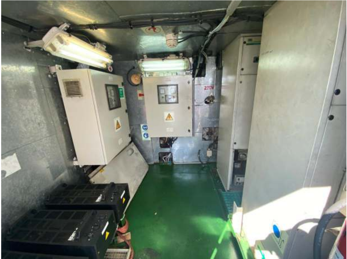
081. Wheelhouse air-conditioning room.
