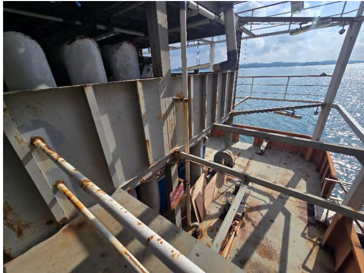
Seawater inlet into filter unit.
