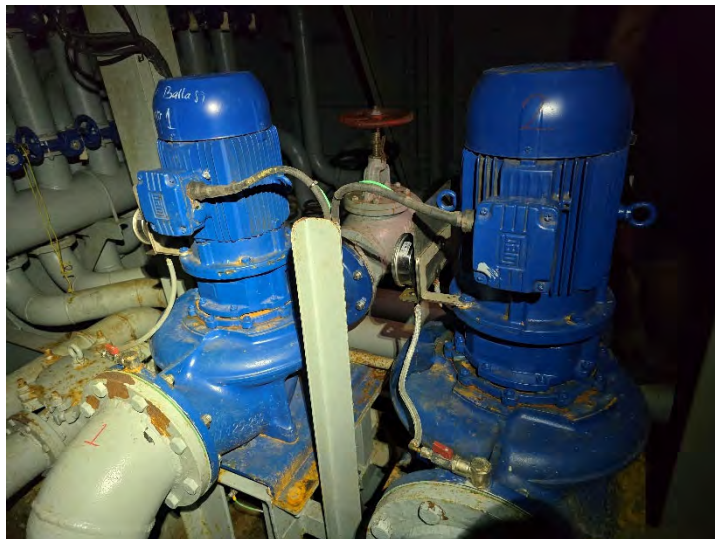
Freshwater ballast pumps.
