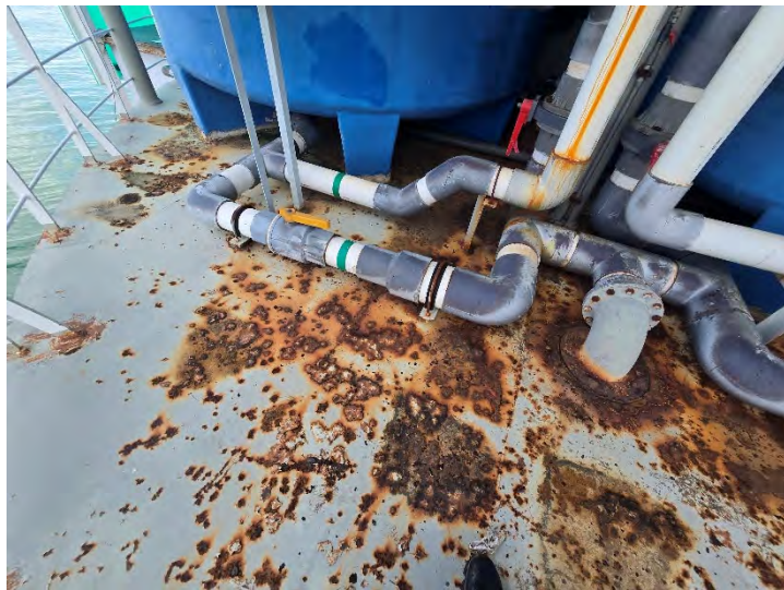
Main deck (aft) plating corroded.
