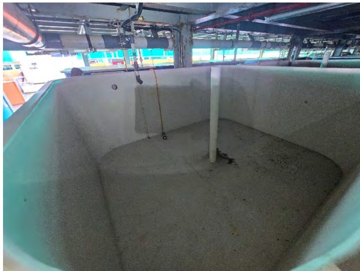
Inside of fibreglass rectangular tanks.
