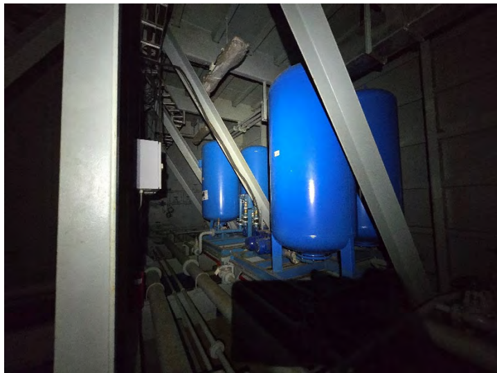
Freshwater hydrophore tank and pumps x 4 set.
