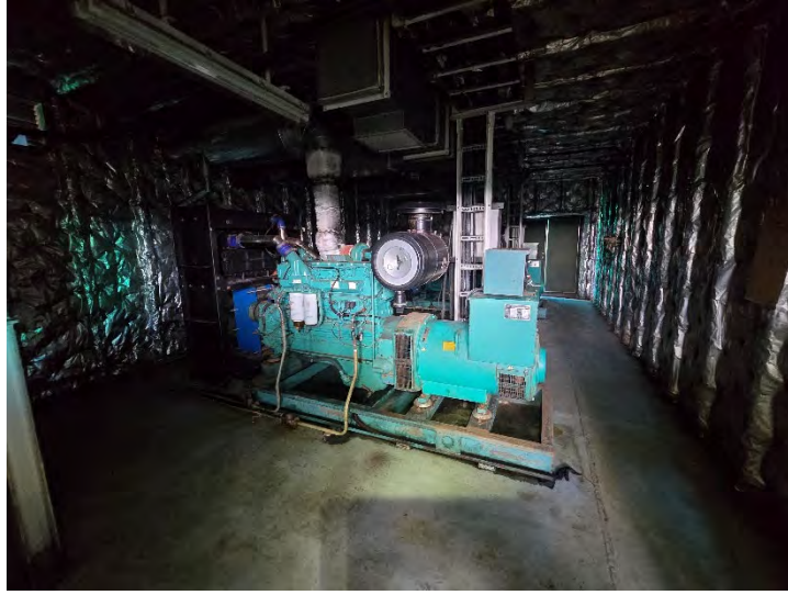
Aux. engine room.
