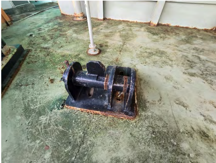
Close up of towing bracket corroded state.
