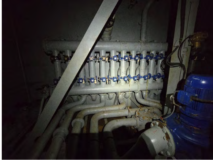
Ballast valve manifold.
