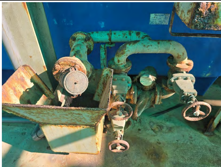
Diesel oil bunkering manifold.
