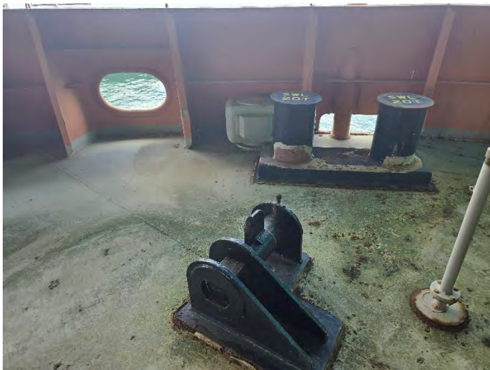
Towing bracket and double bitt on forward deck port found with corroded foundation welding seams.
