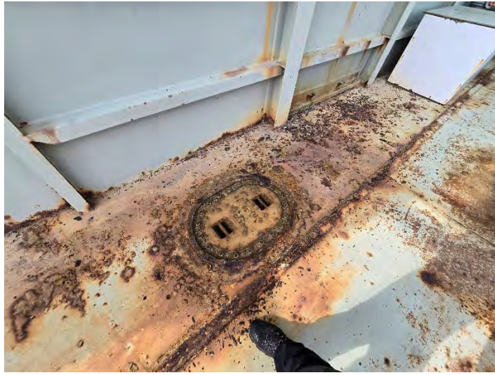
Rusted main deck plating.
