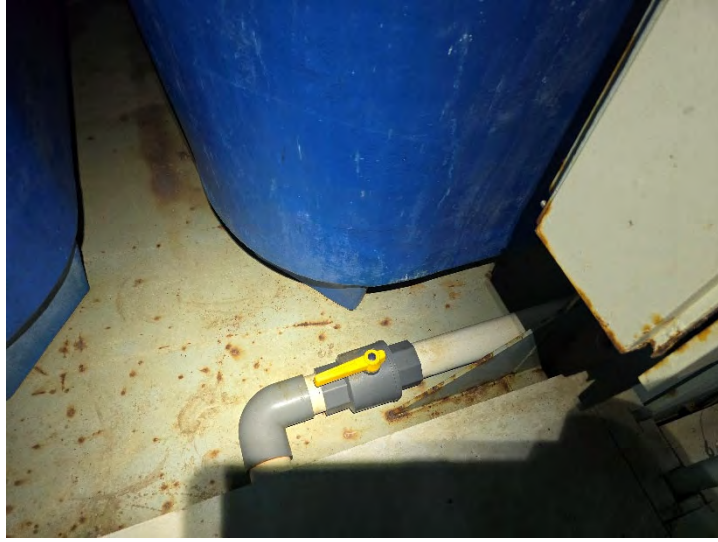
Drain valves for tanks.
