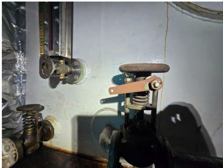
No quick closing valve remote activation wire connected to release mechanism.
