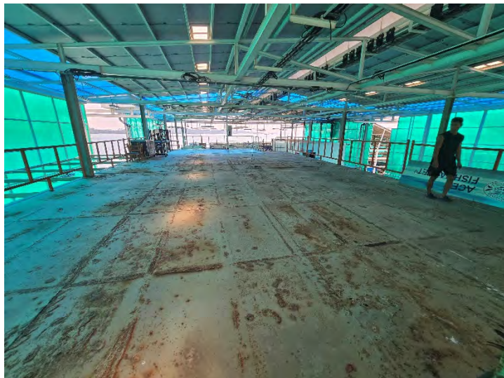
Bridge deck plating in corroded and blistered state.
