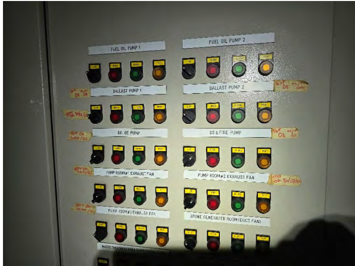
Auxiliary services control panel.
