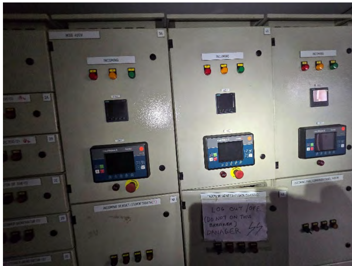
Aux engine switchboard panels.
