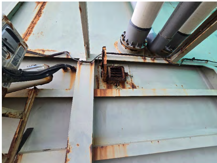
Ventilation flap for farm office wasted.
