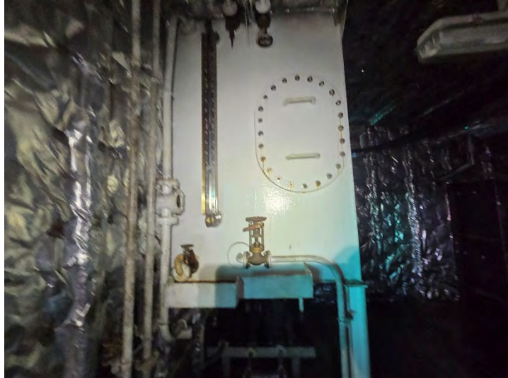
Diesel oil service tank for aux. engines.
