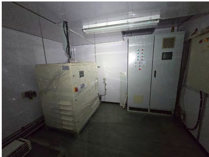
Ozone room with ozone generator and master control panel.
