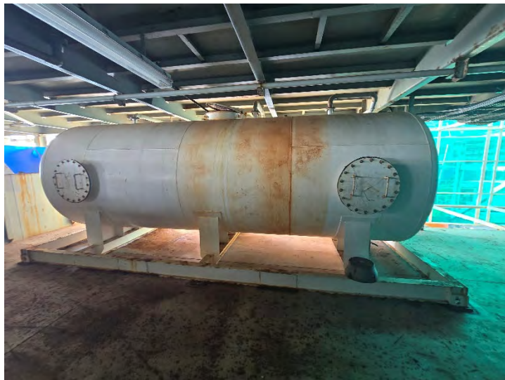
Aux. engine jacket cooling tank.
